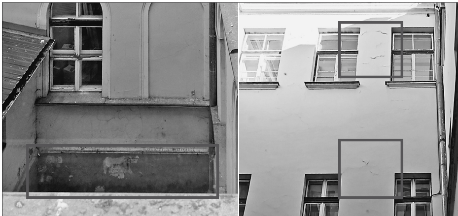
FIG. 6 MOISTURE PENETRATION, CRACKING, AND PEELING OF THE MATERIAL (AUTHOR'S PHOTOS)
