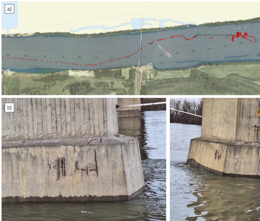
Figure 5. a) Vessel trajectory ; b) damaged bridge column [29]
