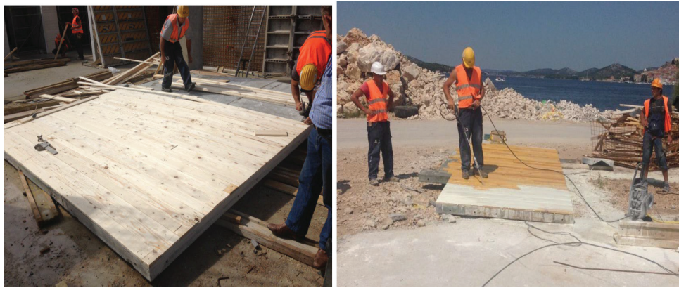
Fig. 8: Preparation of formwork for concrete casting (left) and coating of formwork prior to concrete casting (right).
