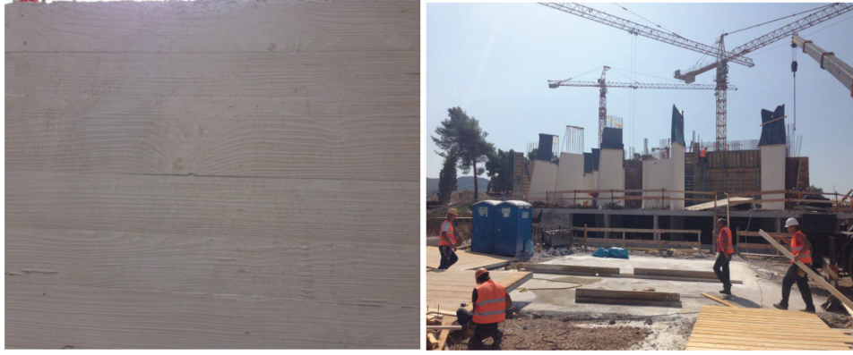
Fig. 7: Final appearance of white concrete walls (left) and view of the hotel during the construction phase (right).
