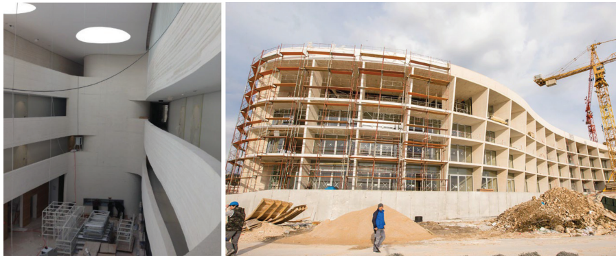
Fig. 9: Visual appearance of the interior (left) and exterior (right) part of the hotel during construction works.
