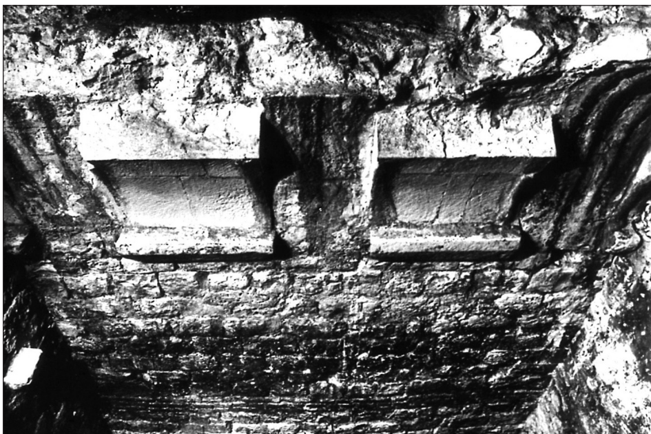
Figure 6. Remains of a bridge-tower, interior
