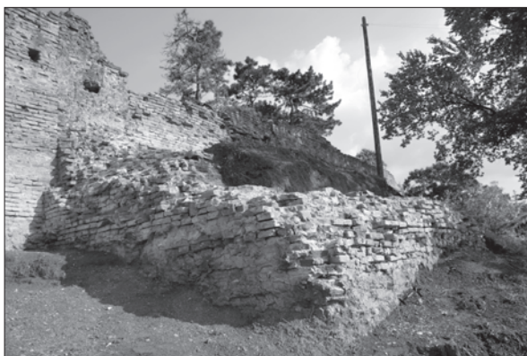
Sl. 14. Zapadna kula, pogled s sjeverozapada (snimio M. Ferenčević) Fig. 14. Western tower, view from the north-west (Photo: M. Ferenčević)
