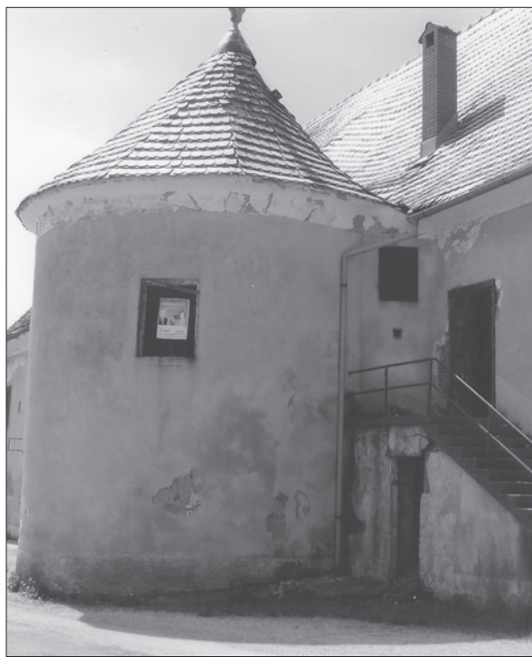
Sl. 1. Sanacija krovišta jugoistočne kule dvorca Mali Tabor (snimila I. Pavišić) Fig. 1. Recovery of the roof of the south-eastern tower of Mali Tabor castle (Photo: I. Pavišić)
