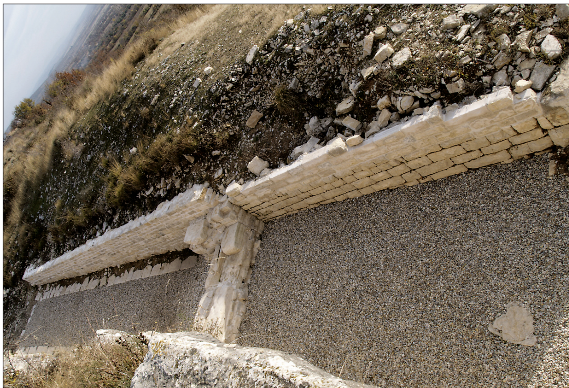
Sl. 7. Pogled na zapadni ulaz s kasnoantičkim pragom - završeni konzervatorsko-restauratorski radovi Fig.7. View of the western gate with the late Roman threshold – after the conclusion of conservation and restoration
