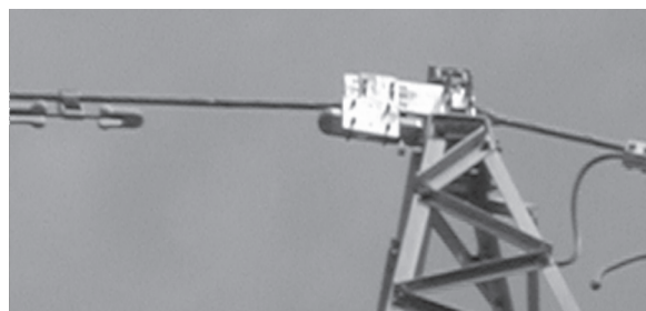
Figure 5. Measuring of aeolian vibrations of transmission line by VIBRECT™ 400
