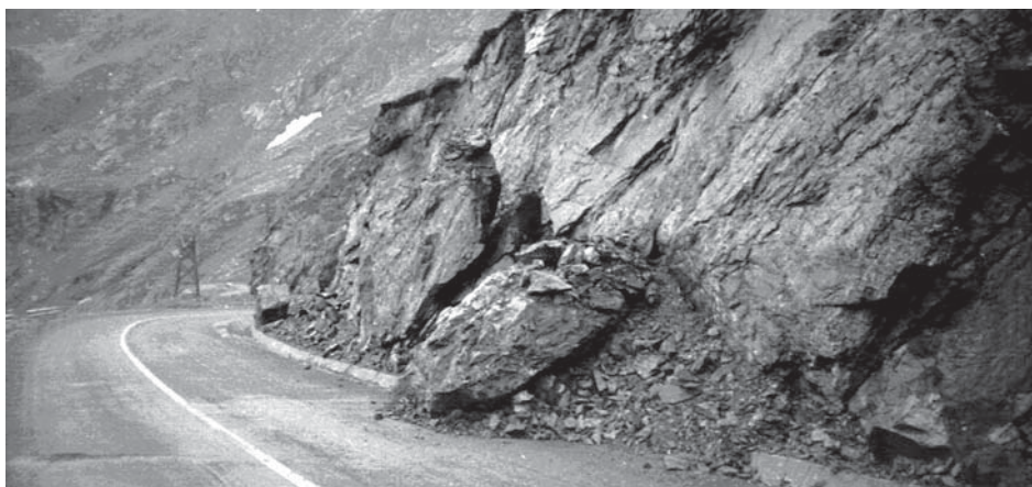
Fig. 5 New cliff, falling blocks and debris on the "Transfăgărășan" road, favoured by the schistosity planes in a typical metamorphic structure
