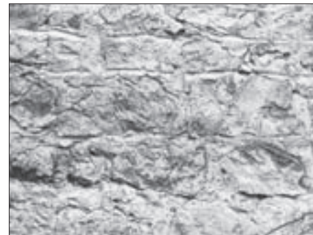
FIG. 7 OKIĆ – GROOVES INSCRIBED ON THE INTERIOR WALL SURFACE, 2 ND HALF OF THE 13 TH C., AFTER EXTENSIONS ALONG THE OLD WALL
