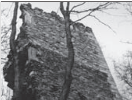
SL. 14. RIBNIK KOD KARLOVCA, NAČIN IZVEDBE LICA ZIDA PETEROKUTNE KULE FIG. 14 RIBNIK NEAR KARLOVAC, PENTAGONAL TOWER, CONSTRUCTION METHOD OF THE WALL FACE
