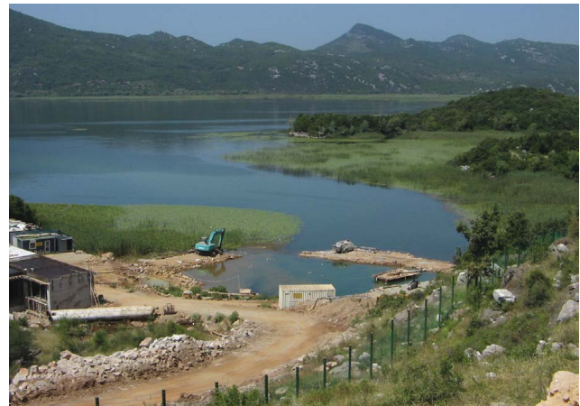
Figure 5: Preparatory works for the foundation of a coffer dam at Bolje sestre spring (STEVANOVIĆ, 2010b).
