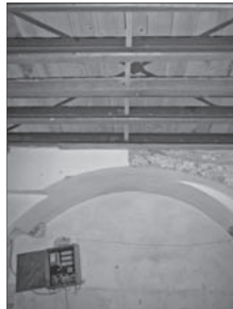
SL. 8. PALAČA U RESTICEVOJ 7, KONSTRUKTIVNO SANIRANA I PRETEŽITO OBNOVLJENA, NOVI STROP PRIZEMLJA FIG. 8 PALACE AT 7 RESTICEVA STREET, STRUCTURALLY REPAIRED AND MOSTLY RENOVATED, NEW CEILING OF THE GROUND FLOOR
