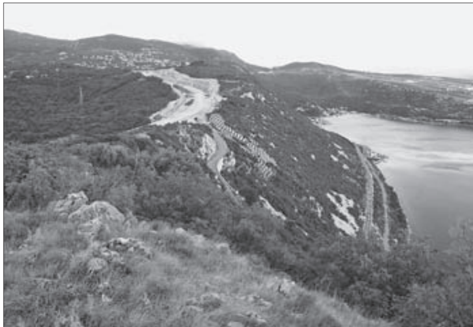
SL. 2. GRADILIŠTE CESTE SV. KUZAM – KRIZIŠĆE NA DODIRU ETNOGRAFSKIH PREDJELA DOLCINA (LIJEVO) I TAKALA (DESNO) FIG. 2 BUILDING SITE OF THE ROAD SV. KUZAM – KRIZIŠĆE, AT THE BORDERLINE BETWEEN THE ETHNOGRAPHIC ZONES OF DOLCINA (LEFT) AND TAKALA (RIGHT)
