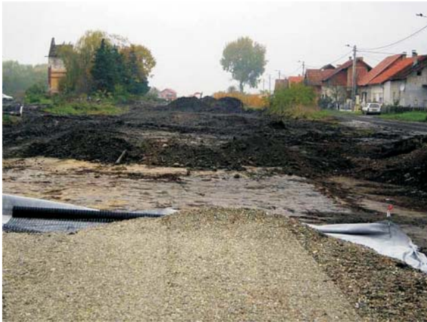
Figure 4 The buffer laid on the subgrade at train stop Antunovac Slika 4. Položeni tampon na trupu pruge kod Antunovca
