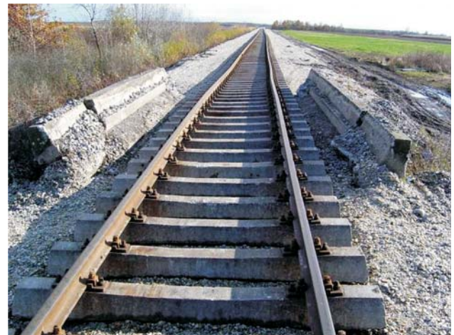
Figure 5 Laid track made of used track materials over water culvert near the train stop Laslovo/Korođ
