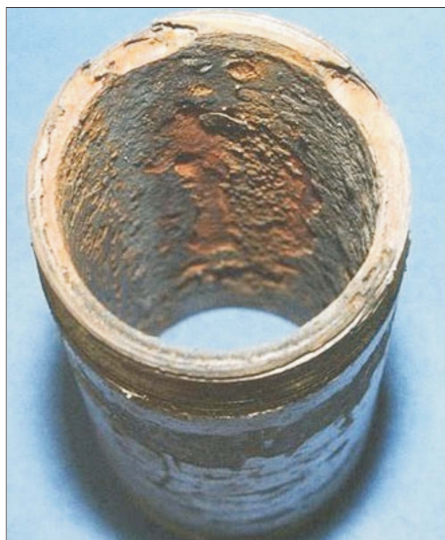
Fig. 4. Image of a metal attacked by crevice corrosions Sl. 4. Slika metala napadnutog pukotinskom korozijom
