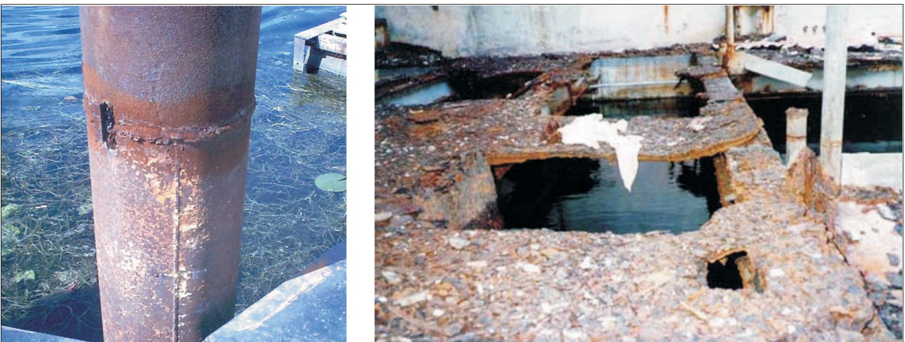
Fig. 9. Uniform corrosion of structural steel
