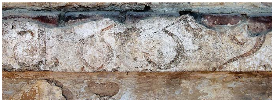
17 Urezana godina 1659. na vijencu između prvog i drugog kata The date 1659 cut into the plaster on the horizontal strip between the 1st and 2nd floors
