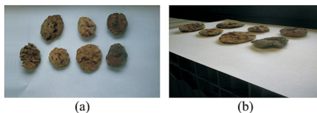
Figure 4 Formed replicas of the largest damages at the bottom of the boiler RP7; (a) The top view: Upper row - Damages at the left hand side end of flange; Lower row - Damages at the right hand side end of flange; (b) The side view
