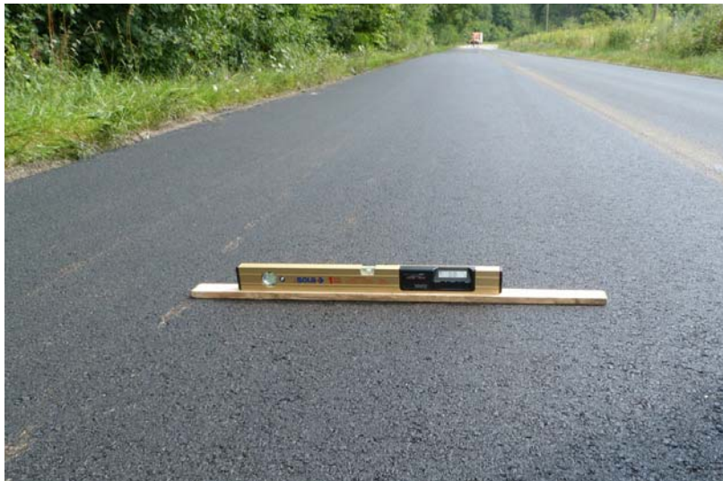
Figure 4. Inclinometer on new layer
