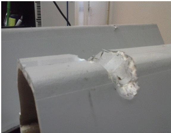
Figure 4. Photograph of beam deformation
