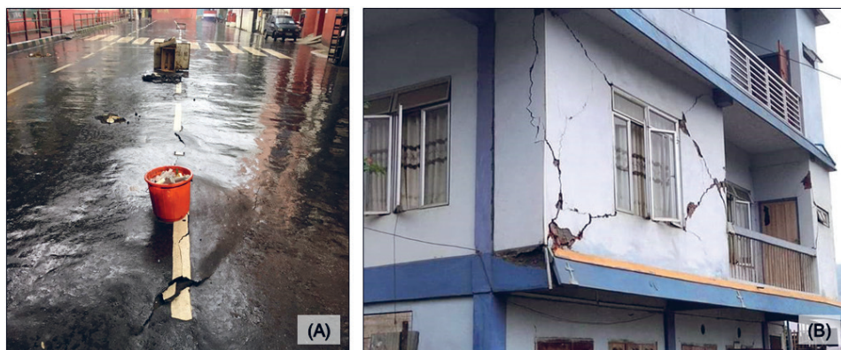
Figure 4. Damages of (A) roads and (B) houses due to 5.5 M_w main shock around Champhai region
