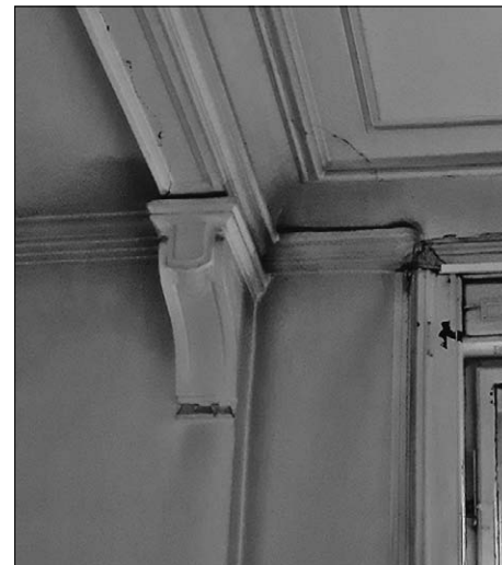
FIG. 9 A DECORATIVE CORBEL ON THE COFFERED CEILING IN THE DIRECTOR’S OFFICE
