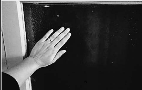
Glass window: cold, permeable, blistered surface (space 2)
