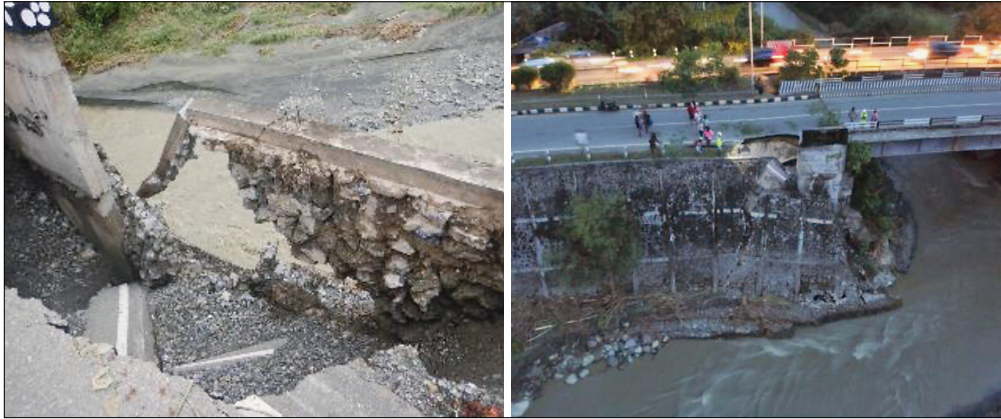
Figure 1: Failure of the bridge abutment structure on the Harapan River
