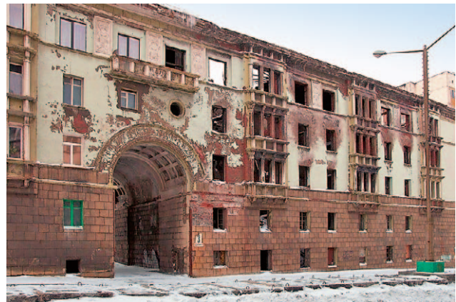
Figure 6: Unfit building at Bogdan-Khmel'nitskiy Street
