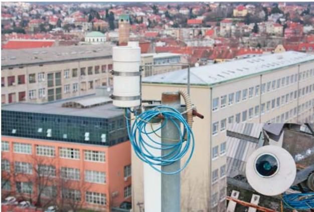
Figure 1: The SQM-LE instrument is mounted on the roof of the faculty building. The instrument itself is put inside a protective box (white) for protection from environmental impacts. The only maintenance required is periodical cleaning of the glass window on the top of the protective box. The inset at bottom-right shows top view of the enclosure, with glass window and the instrument visible inside.
