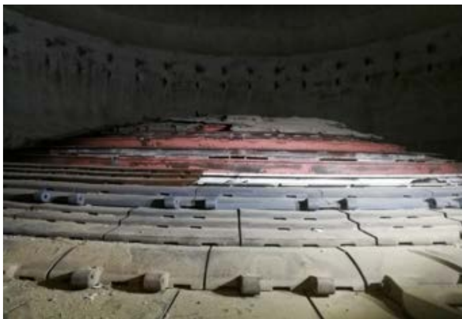
Figure 2. The firebox in the overhaul phase
