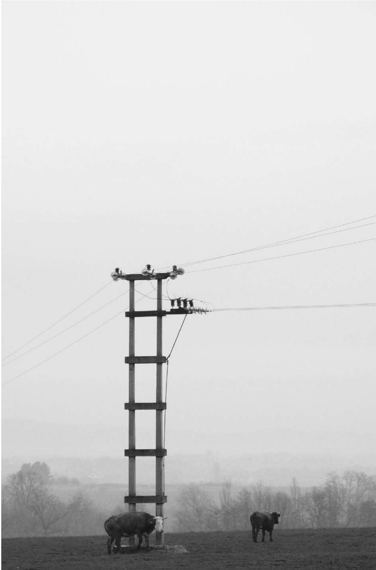
Photo 082. Transmission line / Dalekovod
