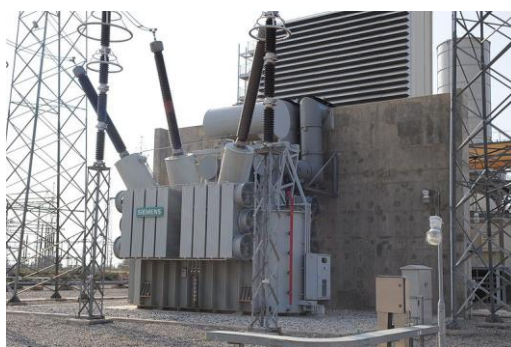
Figure1. High voltage power transformer
