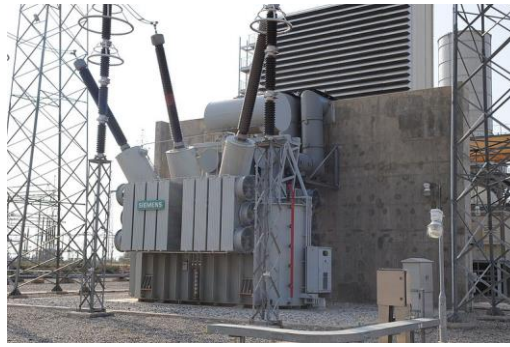
Figure1. High voltage power transformer
